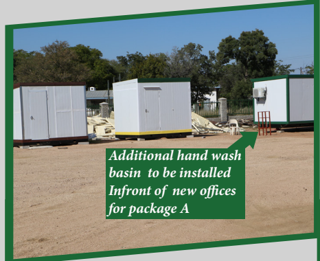
ADDITIONAL PORTA CABINS FOR OFFICE SPACE AT PACKAGE A • Additional 3 porta cabins have been acquired to help to decongest the working space at package A • An additional handwash basin is installed in front of the offices.
