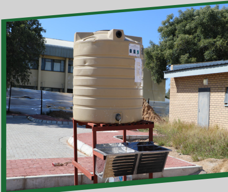
INSTALLED HAND WASH BASIN AT PACKAGE B - PAVED WALK WAY Hand wash basins have been installed at Package "B"- (Hostels and Library). This handbasin is installed next to the paved walk way adjacent to the hostels.
