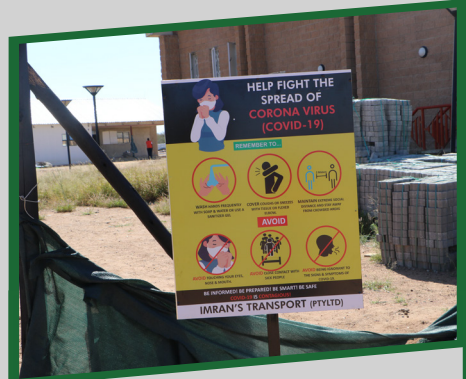
PACKAGE A - ENTRANCE TO SITE SIGNAGE ON COVID - 19 Signage has been improved at the site with COVID - 19 Messages on washing of hands installed at the entrance.
