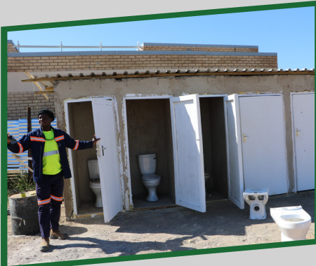
ADDITIONAL STAFF TOILETS being INSTALLED AT PACKAGE "A" Five additional toilets are currently being installed for package "A". This will help to ease congestion and aid social distancing.
