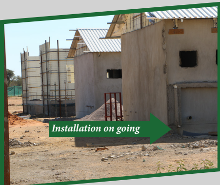
ON GOING INSTALLATIONS AT SCIENCE LABS Additional hand wash basins and elevated water tanks are being installed at the new science labs.
